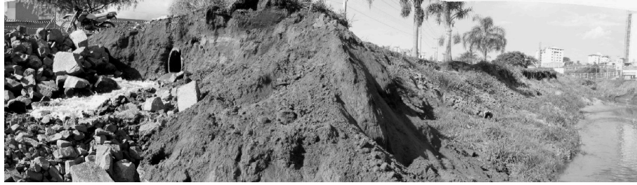
Figure 1: disruption of a wastewater pipeline
