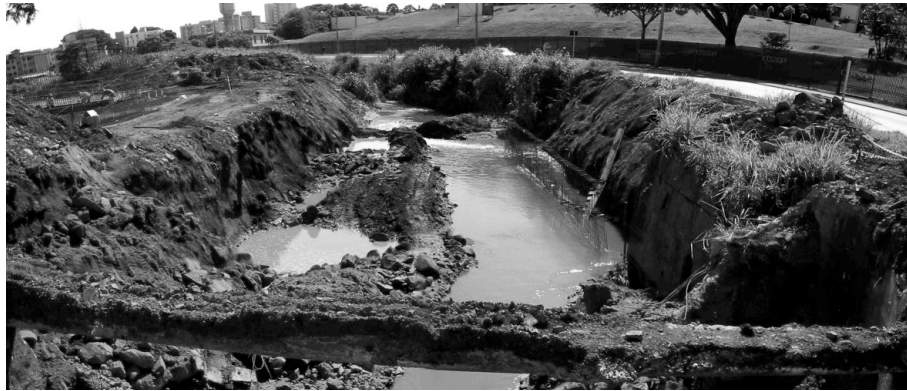
Figure 2: construction of transport infrastructure and impact over Permanent Preservation Areas – soil loss and siltation at urban streams
