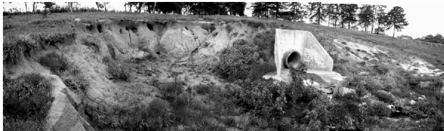
Figure 4: surface drainage equipment causing erosion and degradation in streams
